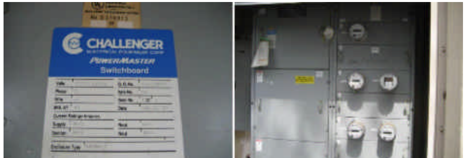
Right building main panel.
